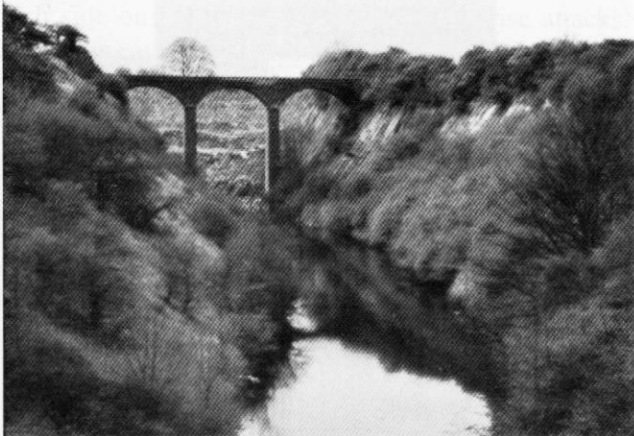
Rain Hall bridge seen from Salterforth Lane (Photo courtesy Mike Clarke). Beyond the bridge the quarry is being filled with rubbish.
